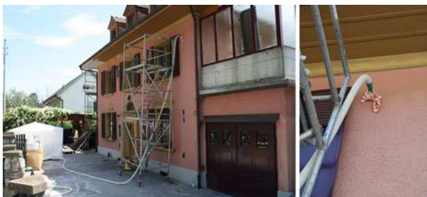
Fig. 20 Cavity wall insulation with aerogel granulate in Biel, Switzerland. View of the renovation site ( left ) and zoom on the injection hole ( right )
