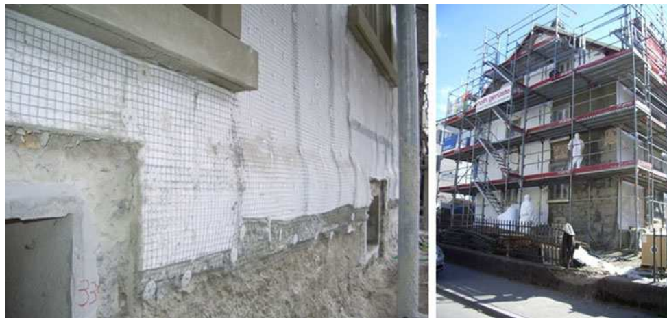
Fig. 24 Retrofit wall insulation with Spaceloft blankets. Wall and window sill detail ( left ) and house side-on view ( right )
