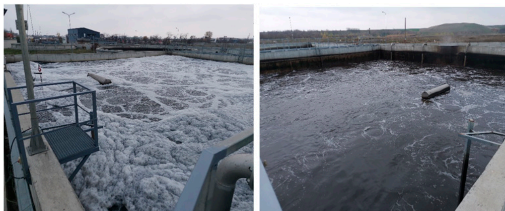
Figure 3. Activated sewage sludge basin (sequential biological reactors).
