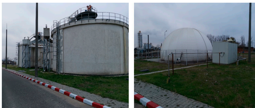
Figure 2. Sewage sludge fermentation tanks (methane tanks) and gasometer. tivated sewage sludge basin (sequential biological reactors).
