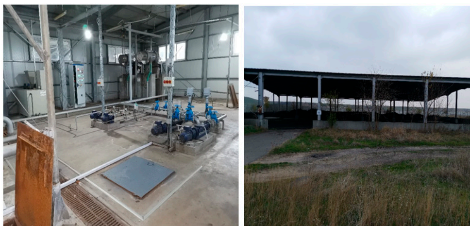
Figure 4. Sewage sludge thickening room (mechanical concentration) and space for the storage of dehydrated sewage sludge.
