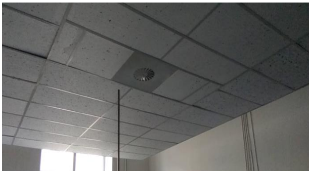
Fig. 2. Diffuser installed in the false ceiling.
