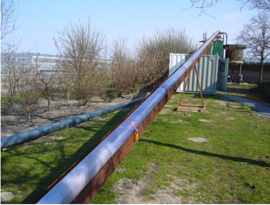
Figure 2: Overview of HvH facility, shown in upstream direction, with the reservoir in the background ( L = 40 m, \Delta z = 7 m, D = 0.192 m)
