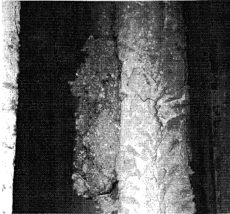
Figure 32 Superheater deposits from Wood-Straw Blend, Grate - 1
