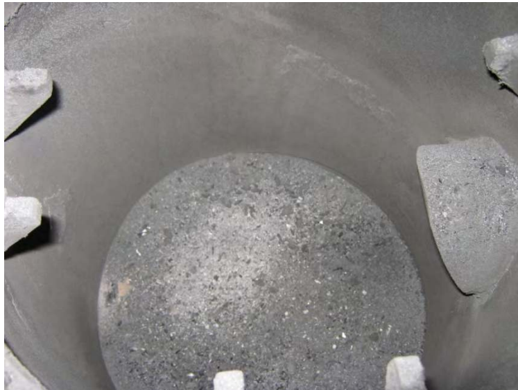
Figure 9-9: Chamber below grate, slanted entrance to tube leading to heat exchanger at right. Larger, heavier ash particles settle here
