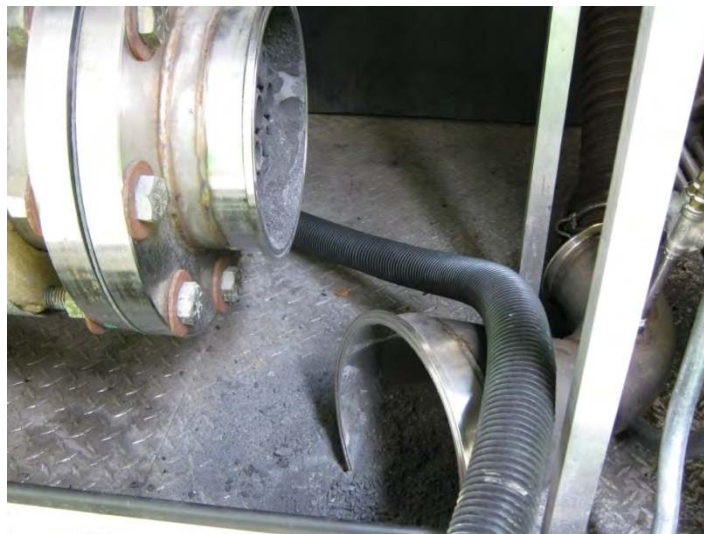
Figure 9-11: Heat exchanger exit, tubes visible inside at left. Pipe bend and flexible hose leading to filter box at right
