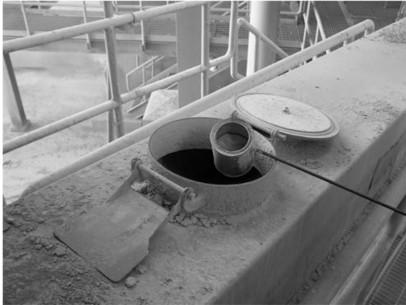
Figure 4-9: Kiln Feed Sampling Point
