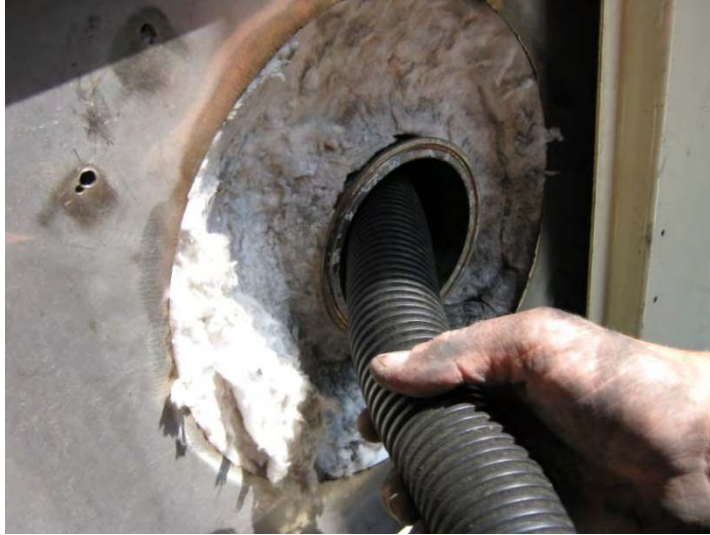
Figure 9-10: Access port at heat exchanger entrance, Shop-Vac in use
