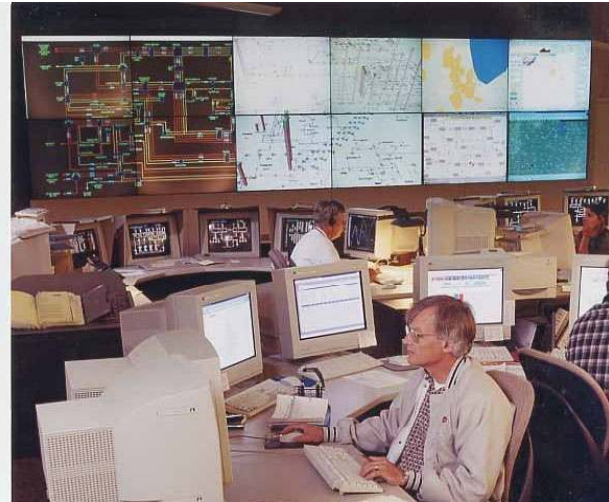
Figure 6: Advanced displays in the control room
