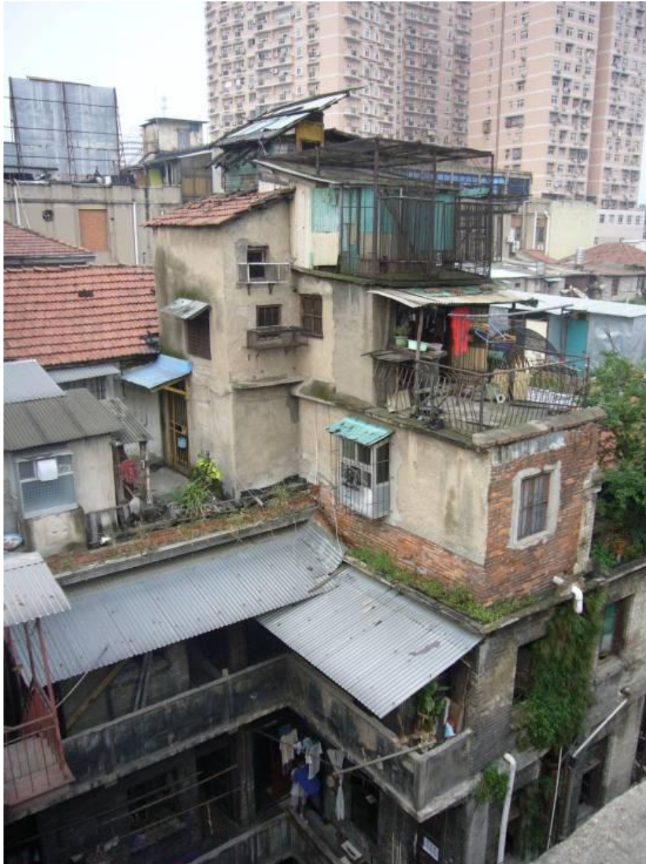
Figure 49 Two or two-and-a-half-storey extensions on the roof have been found on each building
