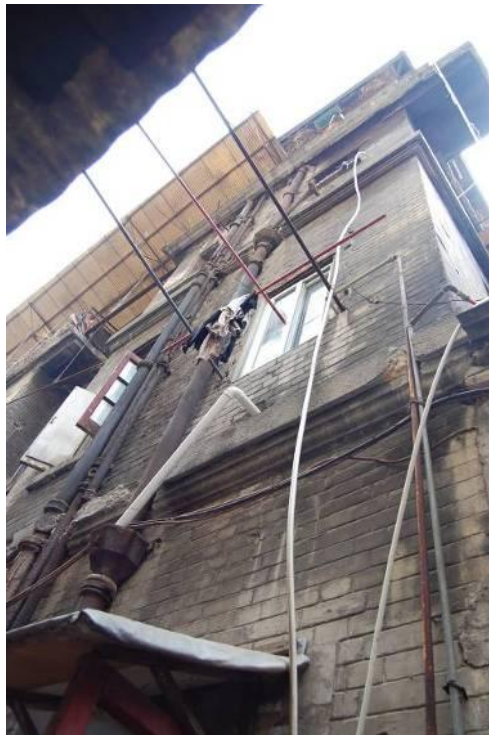
Figure 58 Different pipes and cables made by several households
