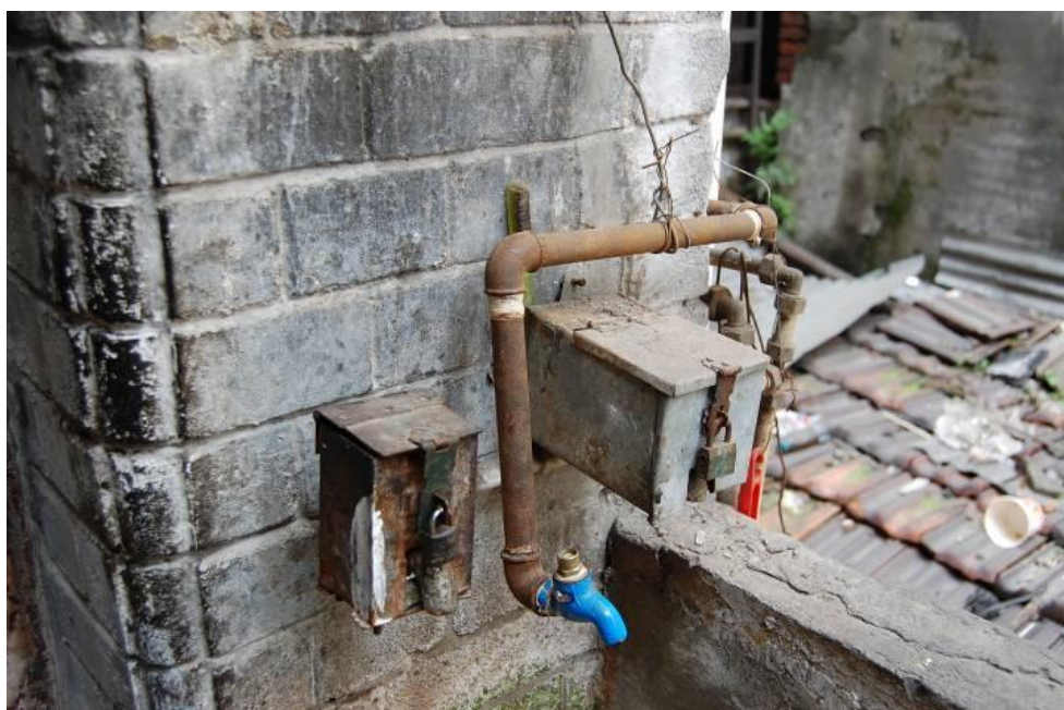
Figure 36 Water taps without head or in locked boxes
