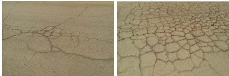
Figure 6.21: Images of this case study: first example of network cracks (block type) (left); second example of network cracks (block type) (right) (UNICOM-UMAP 2014).
