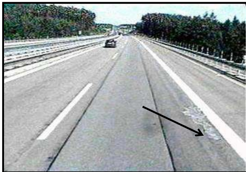
Figure 2.3: Out-breaks (potholes) (FGSV 2006)
