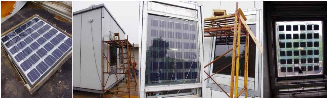
Figure 1: Some of the images have shown the details of the experimental house of BIPV system on the roof of the building. There are two rooms and two windows in the house. Some of the images have shown the details of the photovoltaic panel. There are two different kinds of photovoltaic panels which are installed on the two windows. So a comparative study is possible.
