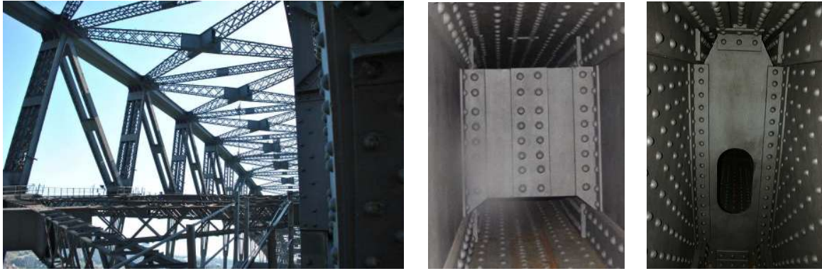
Figure 2: (a) A complex bridge scenario and related difficult areas; (b) a partition plate with limited space on the top and bottom for access and (c) a partition plate with a small manhole for access.
