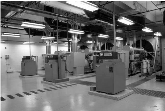
Figure 6: Microsoft Blue Ridge Generator Room
