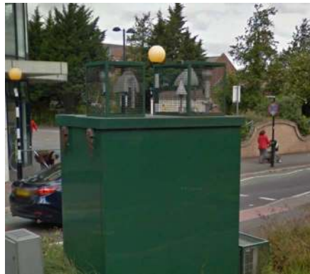
Figure 1: Sensors at Fishergate, York
