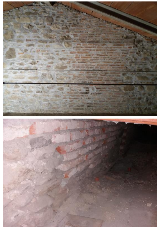
Figure 4. Up: the intermediate wall in the attic where the counter wall supporting the mural painting wall-panel is not present. Down: the counter wall supporting the mural painting wall-panel above the vault but below the attic floor.
