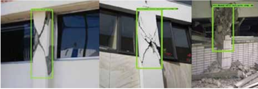
Fig. 6: Bounding box classification results: shear damage to short/captive column
