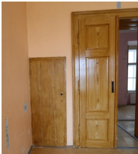
Fig. 12: Nová Horka Castle, room No. 236 with the door leading to the garderobe, photo, 2021 (taken by the author).
