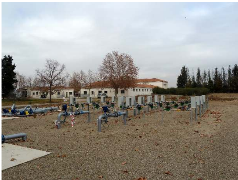
Figure 11: Irrigation system in Aula Dei
