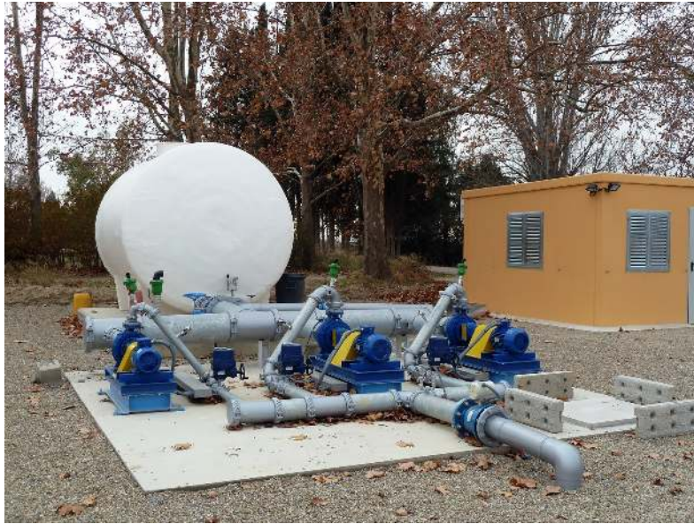
Figure 10: Deposit and three pumping stations in Aula Dei
