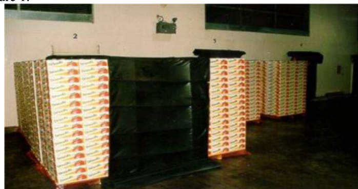
Figure 1: A commercial forced-air cooling system (Source: FAO 2002).
