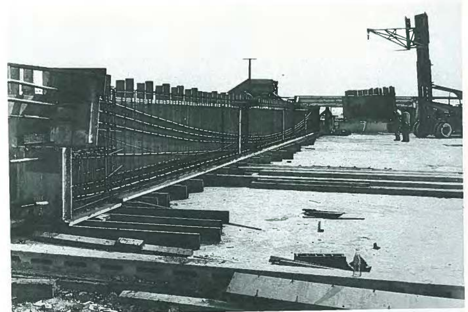
Fig. 76. Formwork for Klickitat County bridge girder showing rubber extractable cores and reinforcing in place prior to casting. Note dividers to separate beam into three segments.
