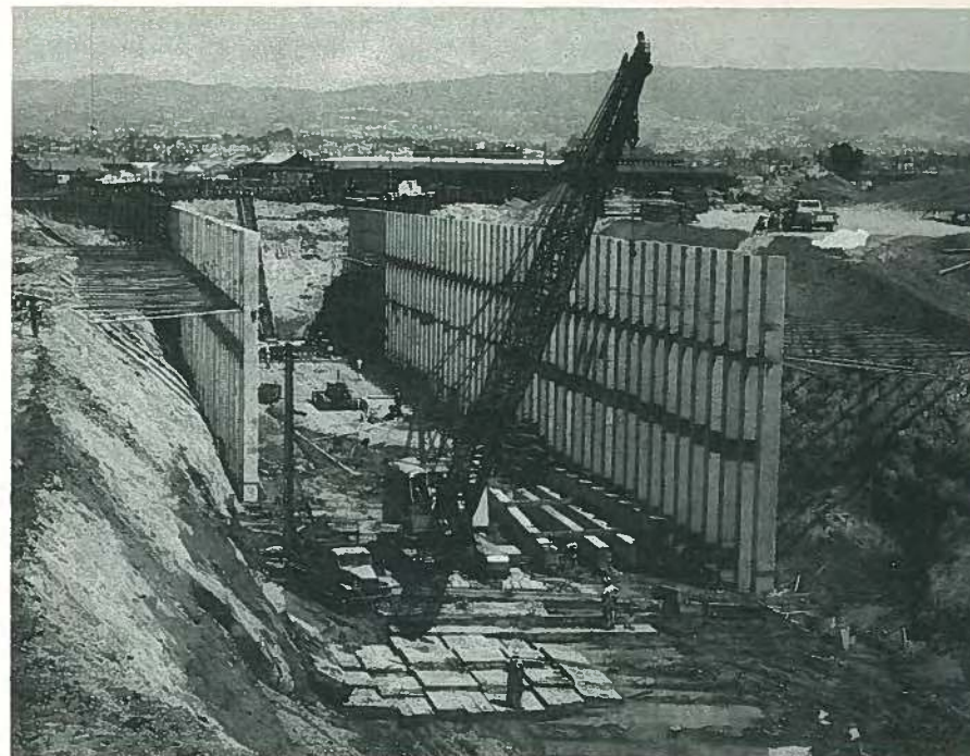
Fig. 54. Contractor's graving dock for manufacture of sub-aqueous vehicular tubes at Webster Street Tube, Oakland-Alameda, California, 1960. Prestensioned concrete soldier beams are designed for maximum negative moments through the addition of mild steel.
