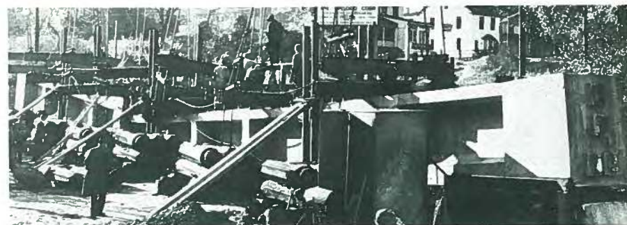
(c) Girder after failure.
