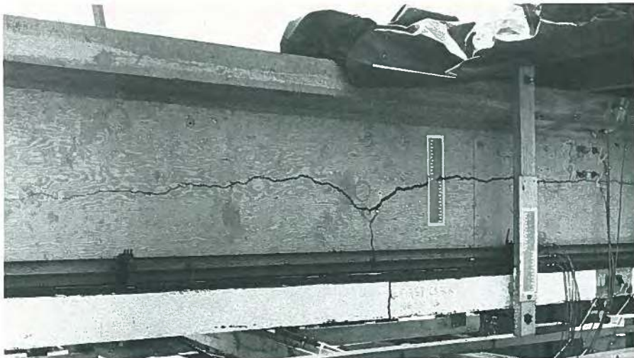
Fig. 39. Crack pattern in 40-ft (12.2 m) prestressed girder (P-40) using external unbonded tendons. The crack originated at midspan at bottom flange running up to the centroid of the girder and then branching out horizontally because no web steel was provided (Austin Company tests).
