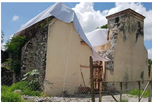
Figure 3. Colonial church damaged by the 2017 Puebla earthquake in Jotutla de Juárez, Morelos. Photo: Adrià Sánchez Calvillo (2018).
