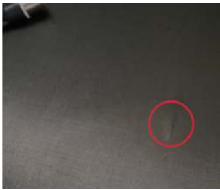
Figure 7. 15mm visible crack present on panel 4
