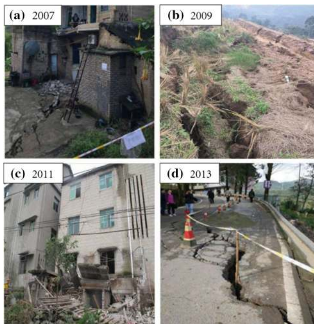
Figure 4. Surface deformation characteristics.
