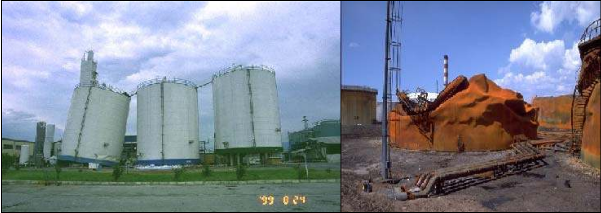
Figure 21a-b. (a) Sloshing damage to upper shell of tank (left), Elephant-foot buckling of the tank wall. (b) yielding of the support structures (left), collapse of the tank (right).
