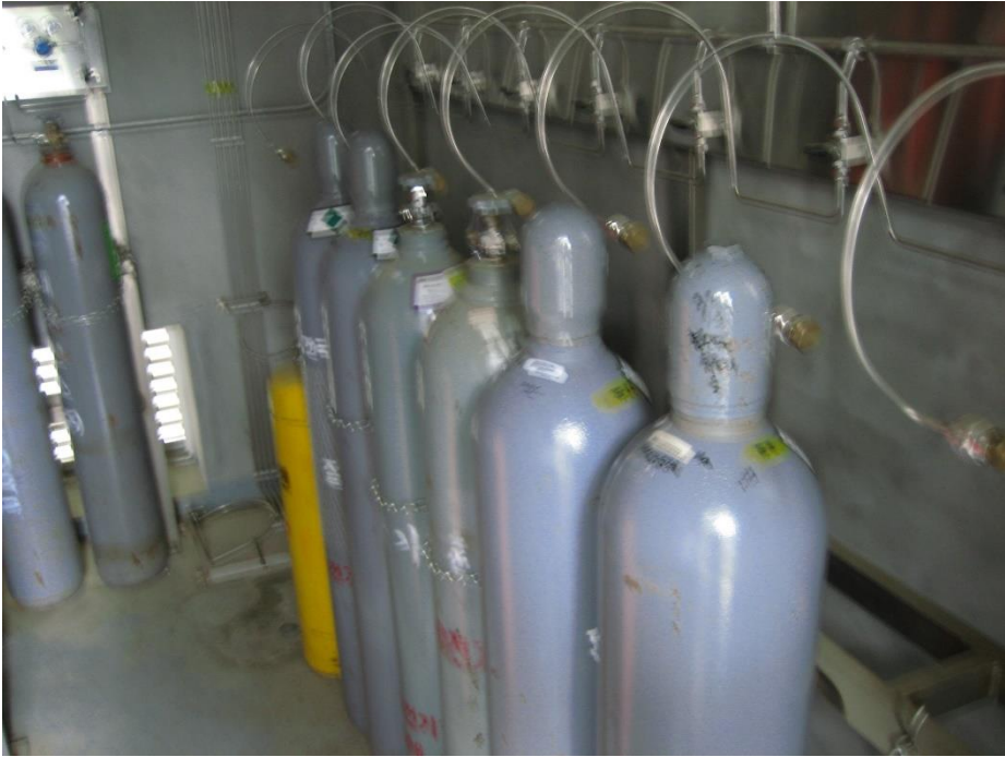
Fig. 3.4. Compressed air tanks.
