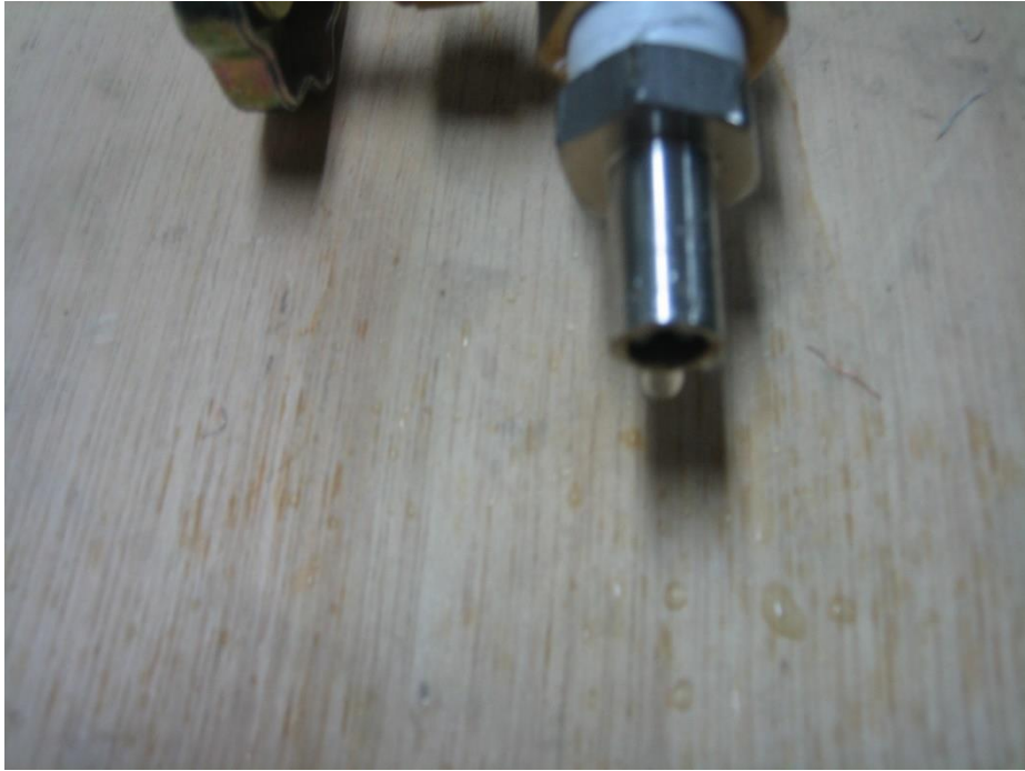
Fig. 3.21. Condensed water at the ejector exit.
