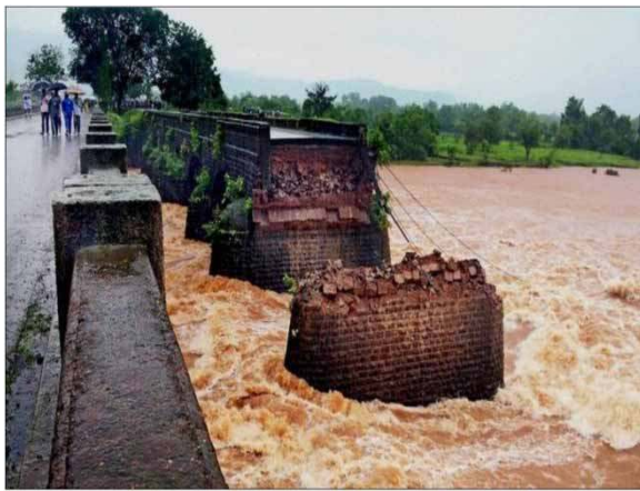
Figure 1 | Collapsed Bridge, Mahad. Source: timesofindia/bridge-collapse-on-goa/liveblog .
