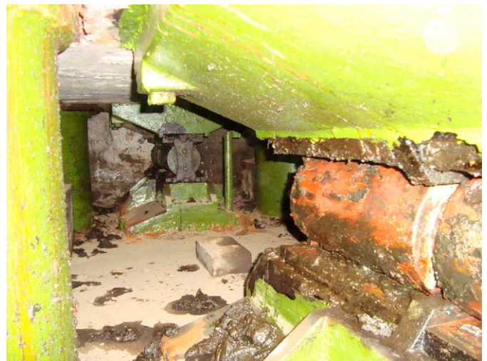
Fig. 3. Roller bearings supporting a bridge pier (image courtesy of Dr. Peter Bennett, taken September 22, 2009)
