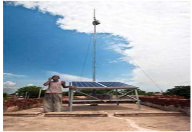
Fig. 6. A Low Powered Cell Phone Solar Powered Base Station [15]
