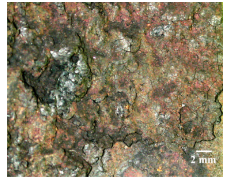
Figure 6: Macrographic analysis. Magnification of a detail from Fig. 4. Corrosion scale.
