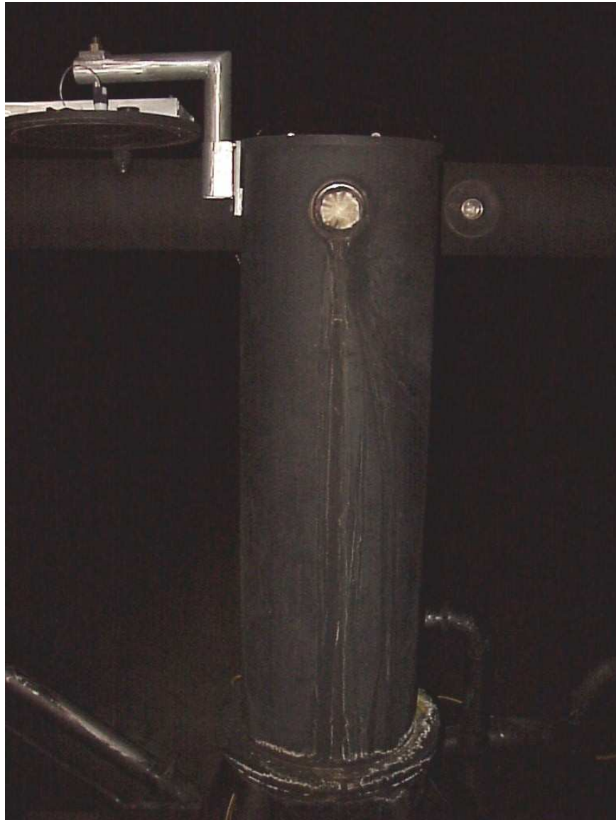
Figure 2.14: Protective enclosure, a cylindrical structure called the periscope, protects the IR camera from the hot exhaust gases and vibration from the engine. The large circle on the upper half of the periscope is a zinc selenide AR-coated window that is transmissive in the infrared. The small window to the right of the infrared window was used in previous tests for a video camera. In this photo, the top of the periscope is open to allow access to the IR camera. The shiny structure to the left of the periscope is the lid and lid support-arm.
