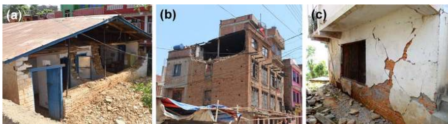
Fig. 3 a URM-SM OOP damage (credit: Suraj Shrestha, EERI photo archive), b URM-BM OOP damage at higher story (credit: Bipin Shrestha, EERI photo archive), c URM-BC IP damage (credit: Bret Lizundia, EERI photo archive) (EERI 2019)
