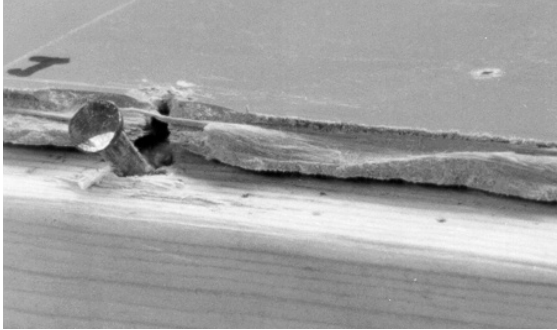
(c) Sheathing cracking
