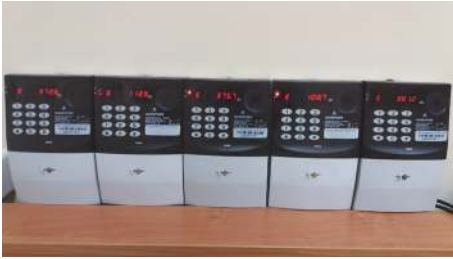
FIGURE 5: Cluster of electricity power meters in building 2.3.
