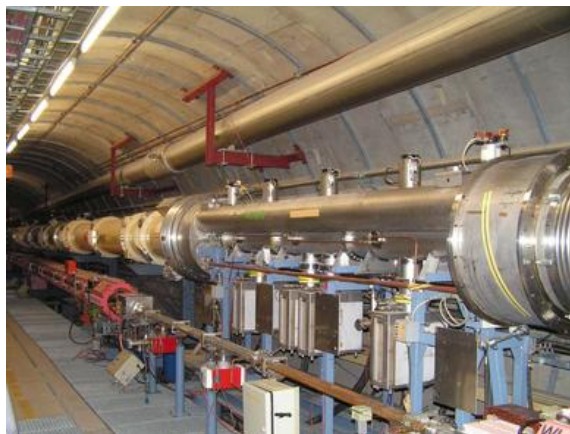
Figure 29. Kicker bypass in the HERA tunnel (West left 200 m). The bypass will be installed in the middle of the experiment connecting the two dipole strings of ALPS-IIc and pass the magnet current and the cryogenics around the optical setup.
