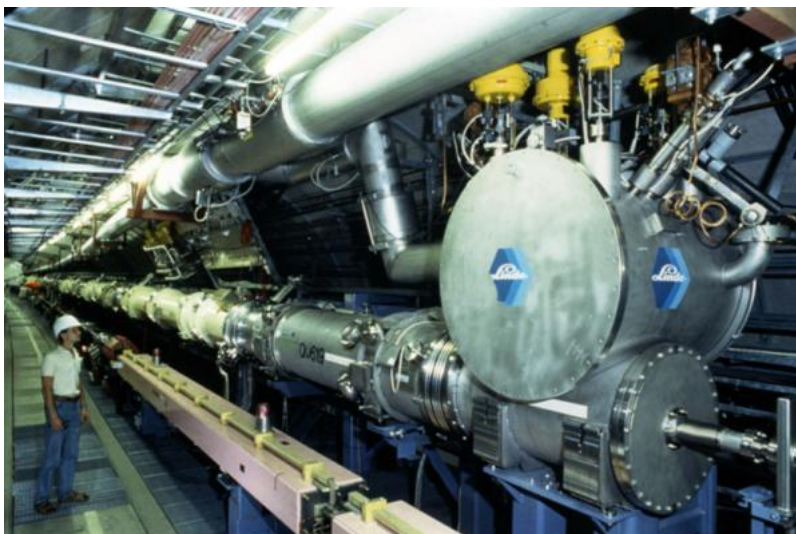
Figure 33. Cryogenic feed box for an octant of superconducting magnets at HERA.
