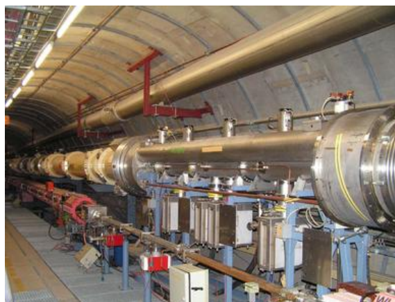
Figure 29. Kicker bypass in the HERA tunnel (West left 200 m). The bypass will be installed in the middle of the experiment connecting the two dipole strings of ALPS-IIc and pass the magnet current and the cryogenics around the optical setup.
