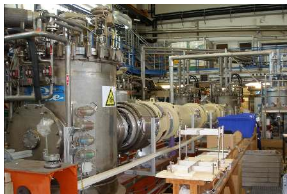
Figure 26. Test bench with the HERA dipole used for the ALPS-I experiment. It is located in hall 55 and will be used to test all dipoles foreseen for ALPS-IIc.
