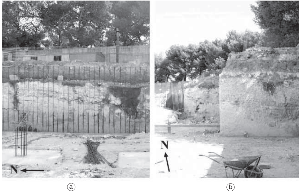
Fig. 12a,b. Photo of the founding pit wall close to zone B revealing the presence of colluvial deposits and fractures in the calcarenite bedrock dipping to the south (a) and east (b).
