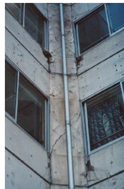
(b) Shear failure of columns
