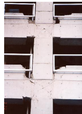
(c) Damage of beam ends and beam-column joints
