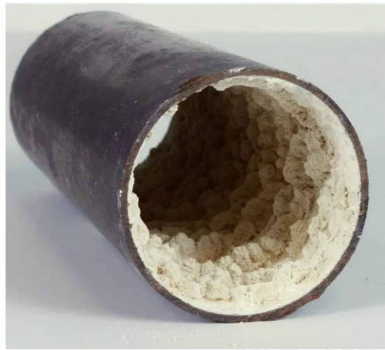
Figure 1. An example of a scale formed in a pipeline.
