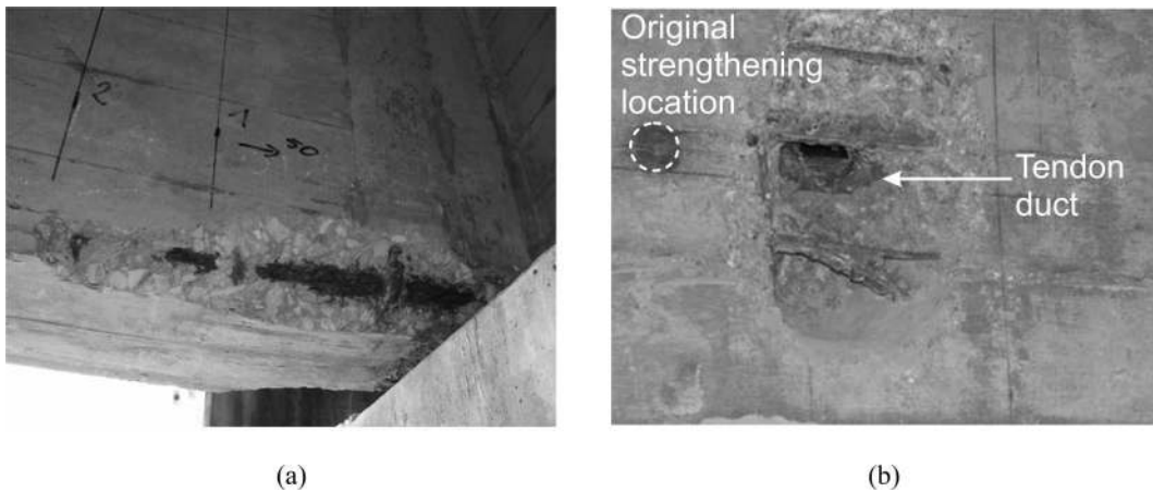
Figure 6. Example of: (a) corrosion of the reinforcement in the Barra Bridge, and (b) window opened in a longitudinal beam for the detection of tendon ducts in the Lanheses Bridge.
