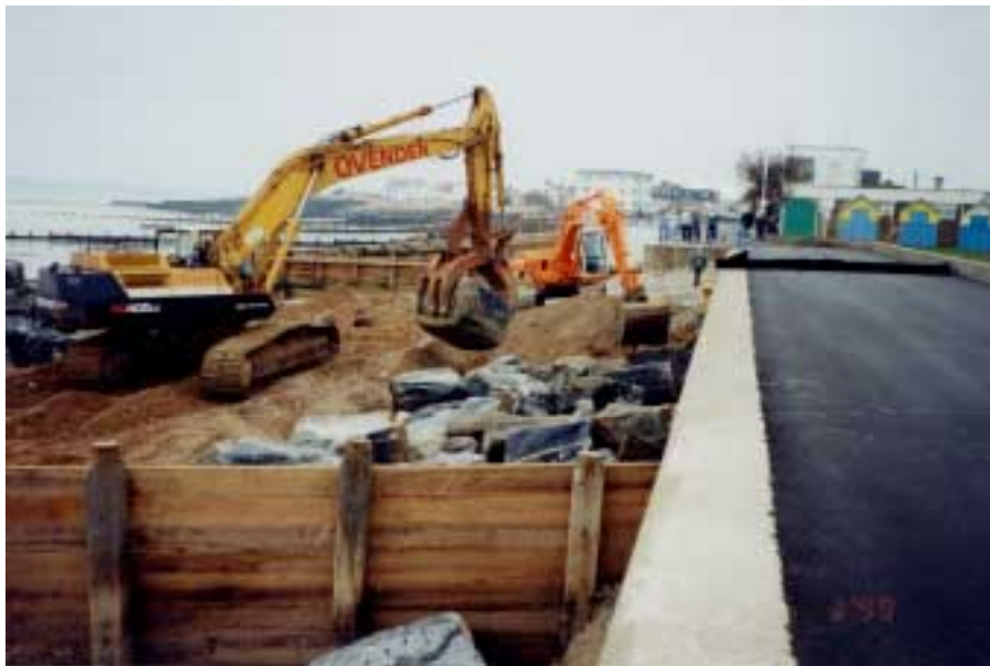
Figure 33. Groynes at Felpham with rock toe in front of seawall (courtesy to Posford Haskoning)
