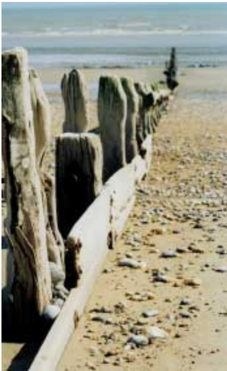
Figure 2. Old and badly maintained groyne (Norman's Bay)
