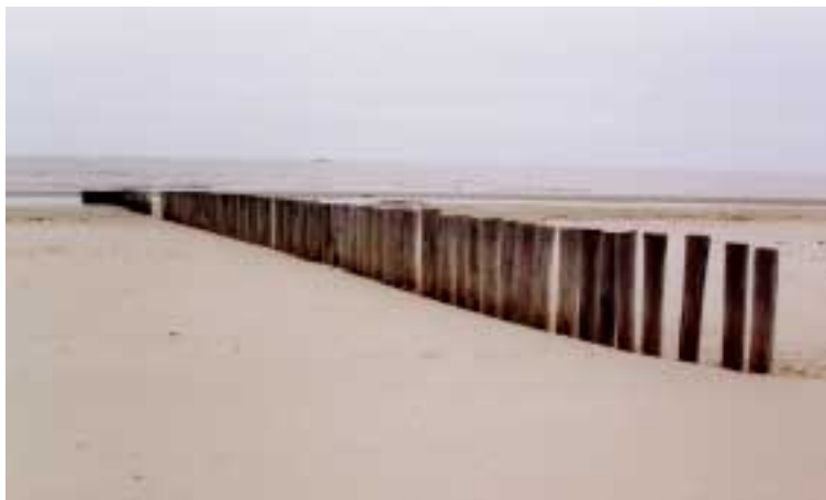
Figure 4. Pile row groyne (Ameland, The Netherlands)
