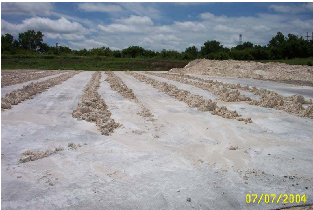
Figure 4: Solar Drying of Sludge in Windrows
