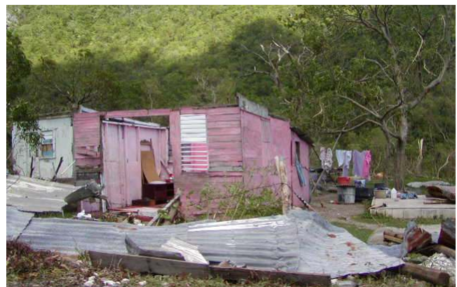
Figure 1. Dwelling in rural Jamaica damaged by hurricane Ivan, 2004
