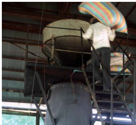
Figure 4. A biomass gasifier in Cambodia generating power from rice husk feedstock
