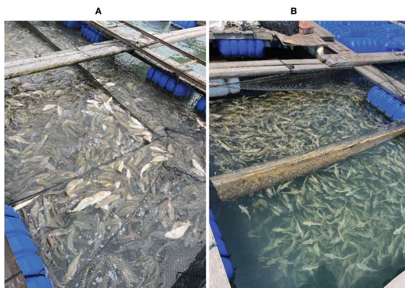
FIGURE 6 Picture of the behavioral response of the large yellow croaker at the range of 598 m for impact pile driving (A) and at the range of 717 m for vibratory pile driving (B) at the beginning of pile driving.
