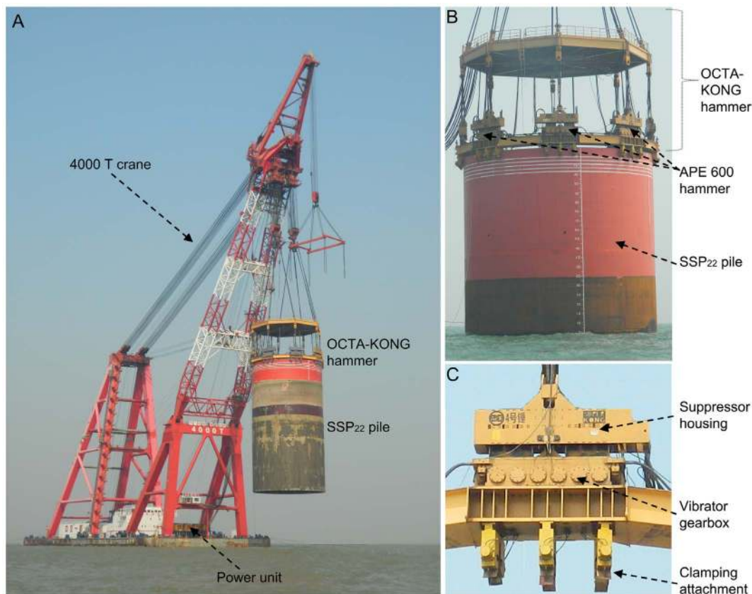
Figure 2. OCTA-KONG vibration operation. During vibration, the pile and hammer are rigidly connected (A). The OCTA-KONG was a tandem combination of 8× APE 600 (B), with each APE600 composed of a suppressor housing, a vibrator gearbox and a clamping attachment (C). doi:10.1371/journal.pone.0110590.g002
