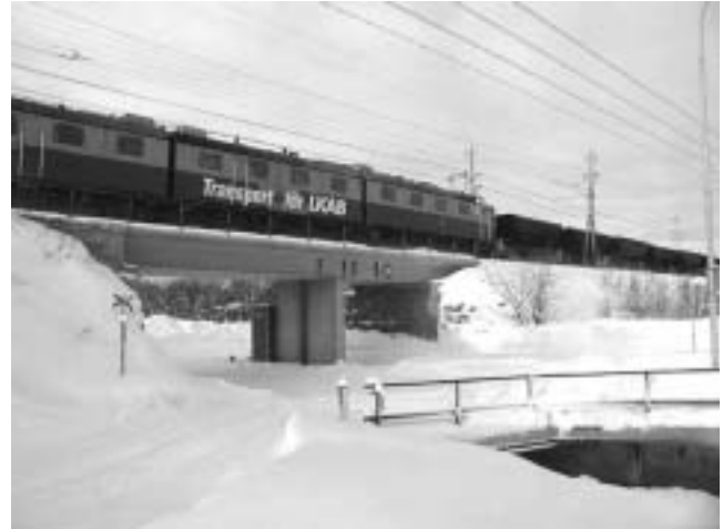
Figure 1. Freight train carrying iron ore over the Luossajokk bridge in Kiruna in the northern parts of Sweden. The bridge is going through an assessment procedure to check its capacity to carry axle loads of 300 kN instead of the present 250 kN.
