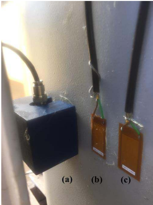
Fig. 4. Sensors installed on the transformer wall: (a) R151-AST conventional AE sensor, (b) MFC-P2 and (c) MFC-P1 sensor.
