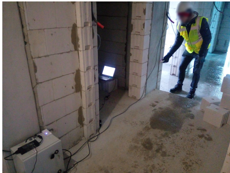
Figure 18. GWEN inside enclosure (bottom left) in a construction site pilot.
