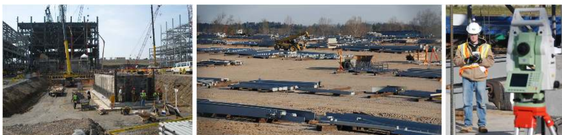
Figure 10 Layout of experiments: construction pit (left), lay down yard (middle), and UWB tag and RTS prism on helmet (right).
