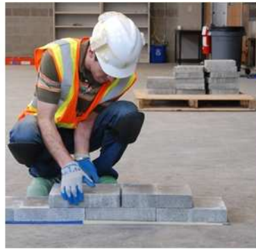
Storage and Installation Areas
