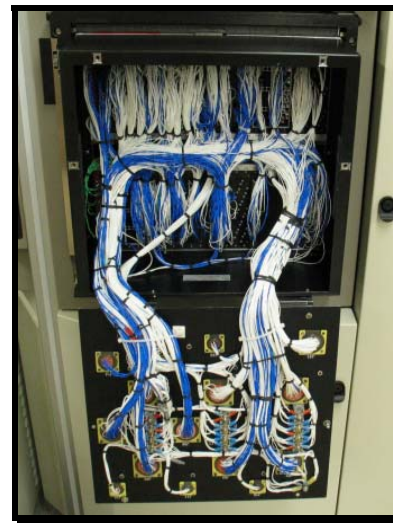
Interface Test Adapter Internal View
