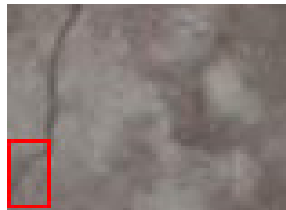
Fig. 5. An invisible crack mark within the rectangular region
