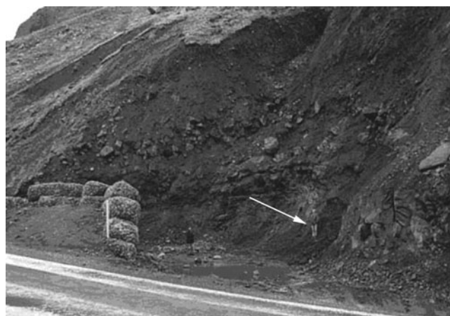
Fig. 5. Catching dam with stack of gabions and location of sensors in path 14.
